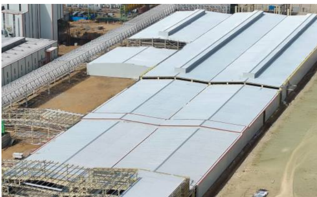
Gwalior, Madhya Pradesh Area: 6.52 Lakh Sqft.
